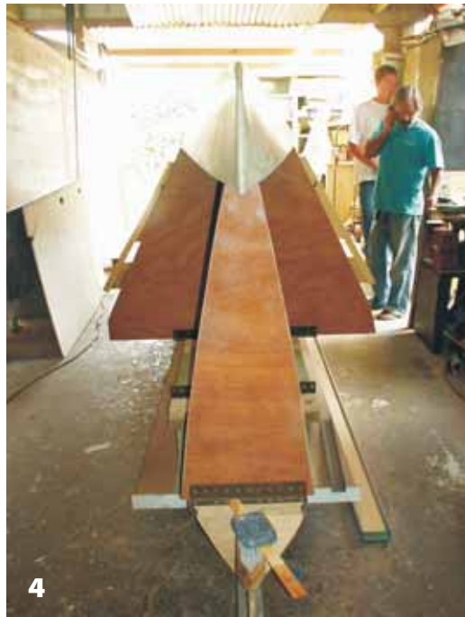
Figure 4—The main hull is built by first attaching bulkheads to a strongback. Here, the pan is glued to the bulkheads before butt blocks are glued to the pan. The topsides are put on last.
