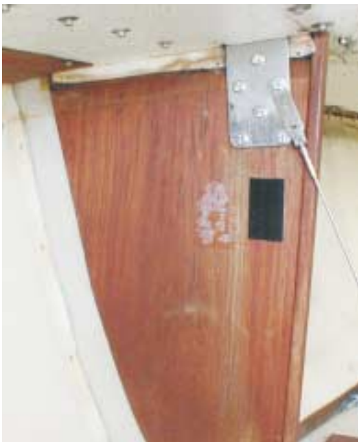
Right—The port bulkhead with the chainplate still attached.
